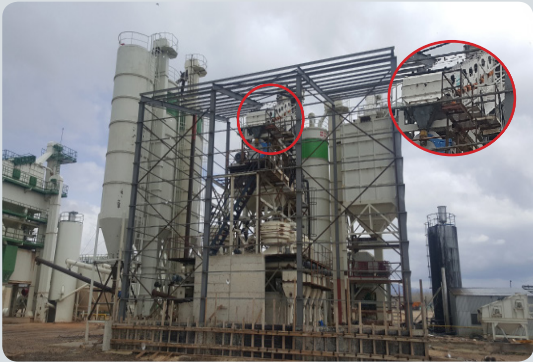
In this plant, a single deck VCR-D screening machine in size of 1500x6000 screens construction chemicals in -0,710 mm with a capacity of 30 tone/hour.
